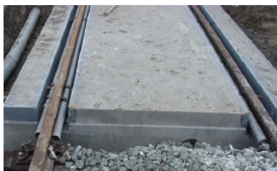
view on installation with PVC tubes
