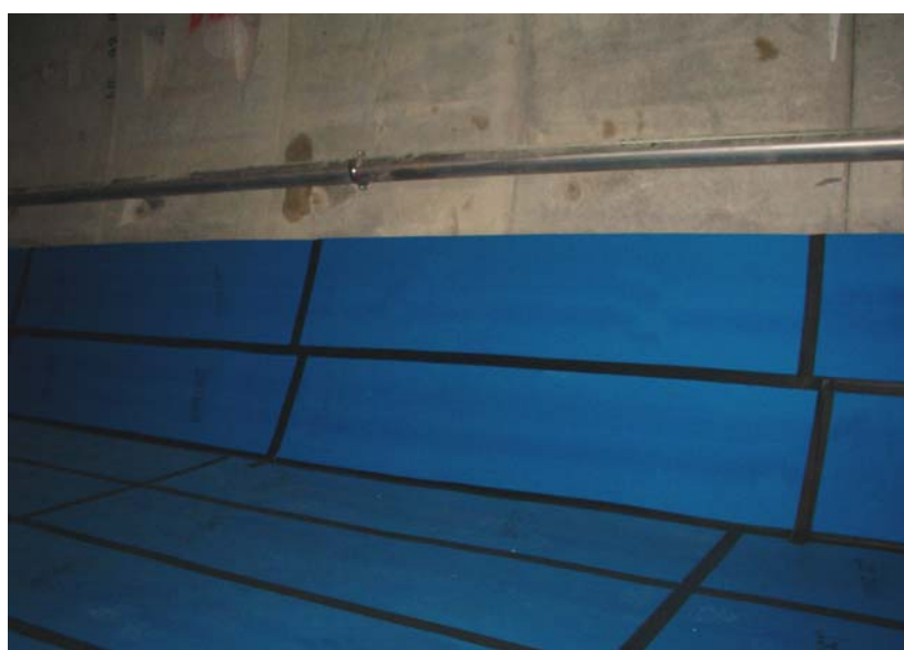
View on the installation of the mat: all joints are well taped off
